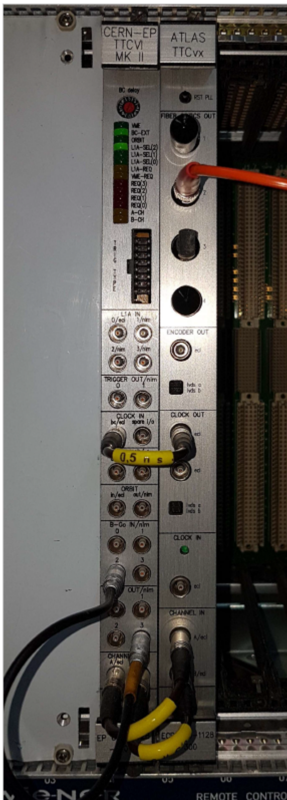
Figure 51. Image of cabled TTC system with B-channel connections
